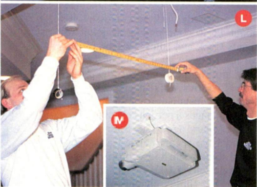
K. Cook secures the video-projector mount to the ceiling using a lag bolt and six screws. L. Cook and Julius use an improvised plumb line to find the center of the 100-inch screen. M. The Sharp XV-S55U LCD projector installed and ready to go.
