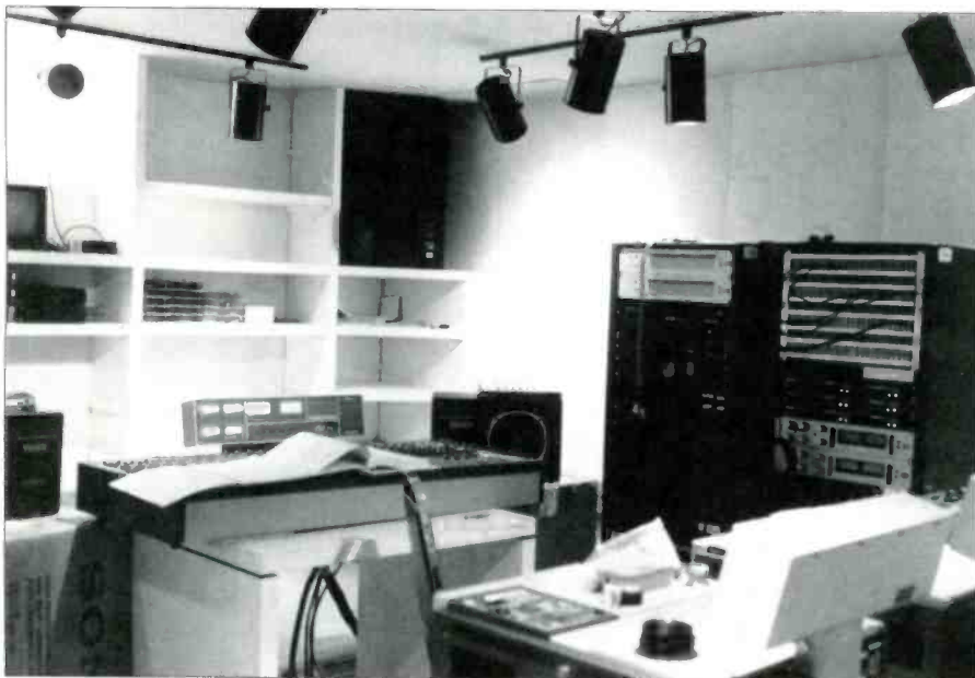
Figure 4. The completed control room with equipment installed.
