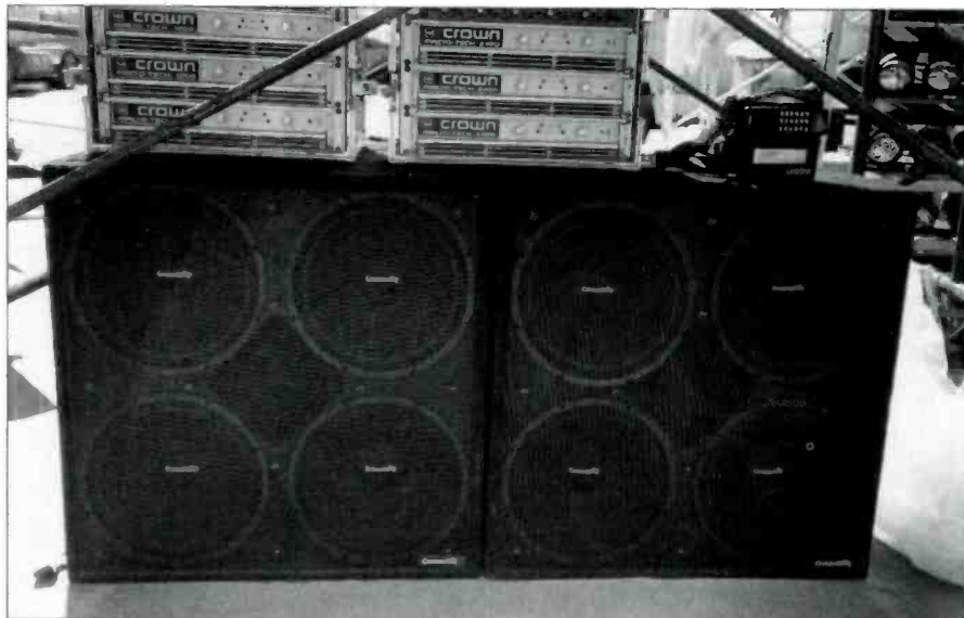
Figure 6. Community Light & Sound's VBS415 Subwoofers installed at the Beach Fest.
