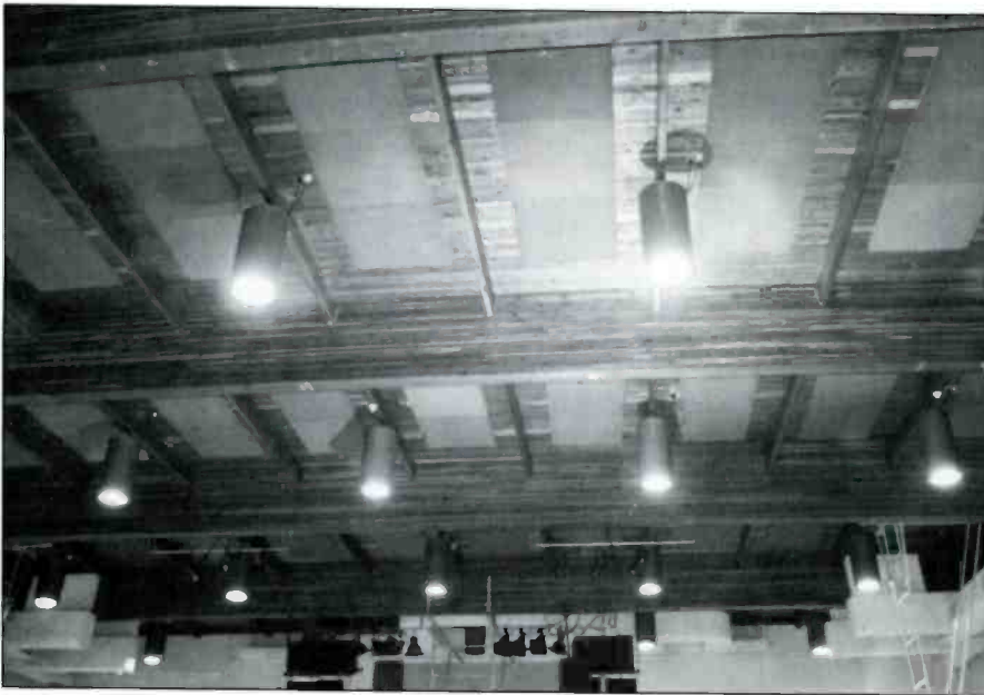
Figure 1. Wedge contoured 3-inch acoustical foam on the ceiling.
