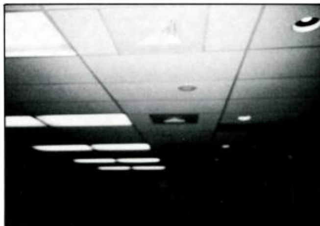
Ceiling showing installation at Health Services Center in Princeton, NJ.
