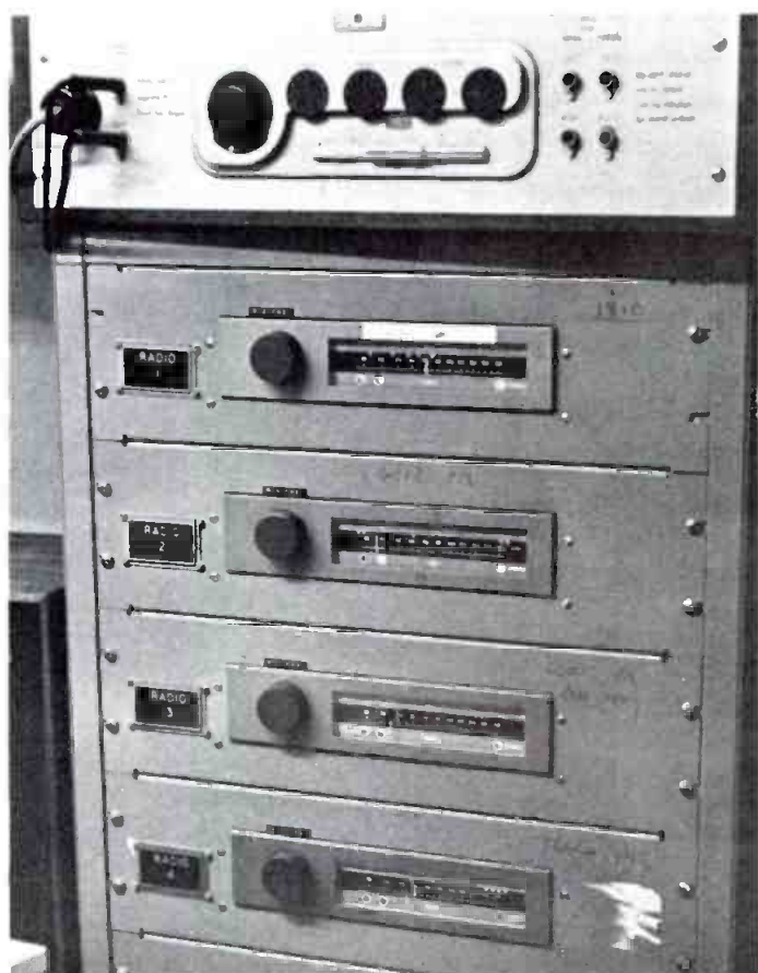
A rack full of quad f.m. tuners for BBC air checks, tied into the automatic time clocks for unattended off-air recording
