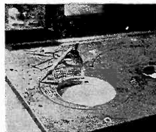
Motor clearance hole was offset with respect to cover-plate outline, and compass was used to find proper position. Compass center is in hole transferred from cardboard template.
