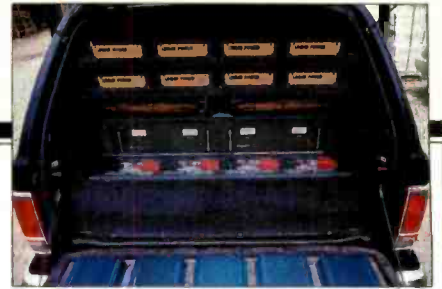
Thirteen amps, five extra batteries, and two a.c. power supplies were used in the Blazer.
