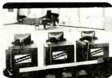
Control-room view of three A-7 Systems used for 3-channel PLAYBACK monitoring at United Recording Studios, Hollywood.
