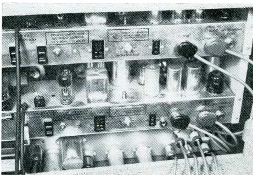
Fig. 2. Rear view shows the very short connections to the tape machine amplifiers.
