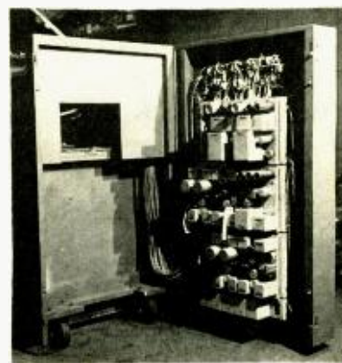
Fig. 5. Second section of the left end opens to permit access to amplifiers.
