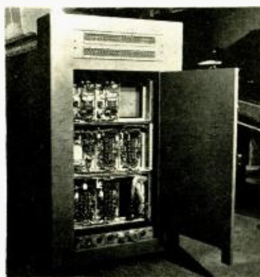
Fig. 4. Left end of the console with the access door open for servicing.
