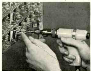
Power tool whips wire on terminal in fraction of a second. There is no heat which could damage miniature components . . . no dropped solder or wire clippings to cause trouble later.
