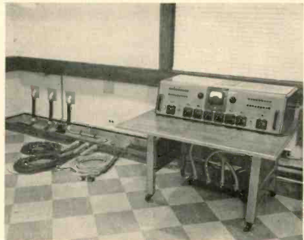
Fig. 1. Stock console in course of installation (RCA Type 76B5). Control room "A" Armed Forces Information School, Fort Slocum, New York. Official Defense Dept. Photo.
