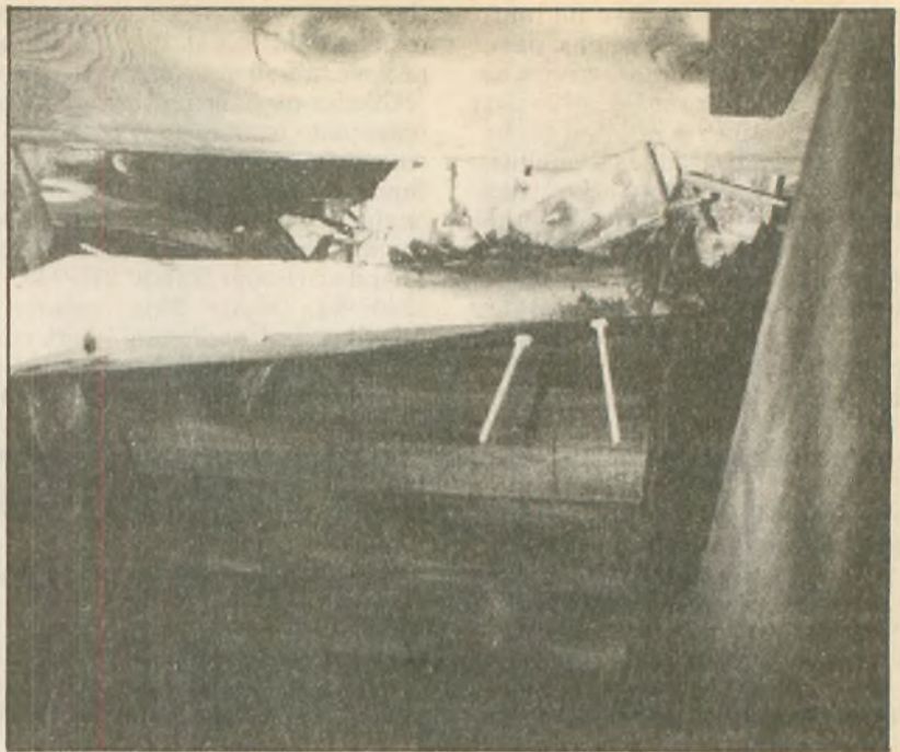
The W2ZEE roof was pierced with fallen antenna tower and equipment.
