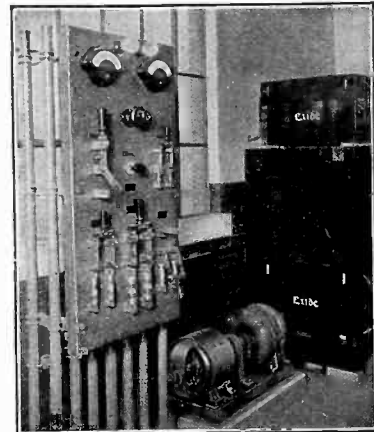
A Diverter Pole Generator floating with a bus control battery in an automatic substation.
