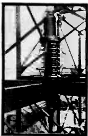
Single Conductor Pothead—Three at end of each cable.
