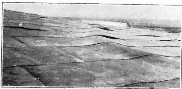
FIG. 1—SHOWING THE EFFECTS ON METAL SHEETS NAILED TO WOOD DECKS CAUSED BY TEMPERATURE CHANGES AND BY FILLING AND EMPTYING THE TANK. IN MANY CASES THE EFFECTS OF CORROSION ARE JUST AS BAD
