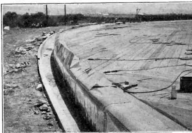
FIG. 10—WATER SEAL FOR THE EAVES OF A LARGE RESERVOIR IN COURSE OF CONSTRUCTION. THE TROUGH IS CONCRETE REINFORCED WITH WELDED MESH WIRE. SHEETS OF ZINC ARE NAILED TO THE DECK AND BENT DOWNWARD INTO THE TROUGH. THE WOOD DECK IS THEN COVERED WITH ROOFING PAPER
