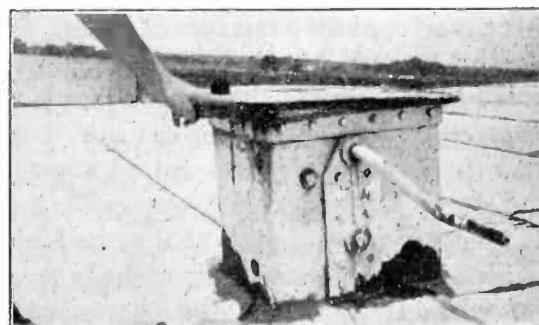
FIG. 4—A WINCH BOX ON THE DECK. THE COVER IS NOT VAPOR TIGHT
