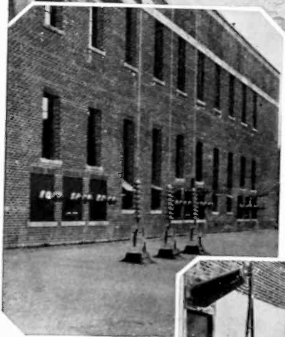
Line entrances at La Gabelle station. O-B suspension insulators and entrance bushings throughout.
