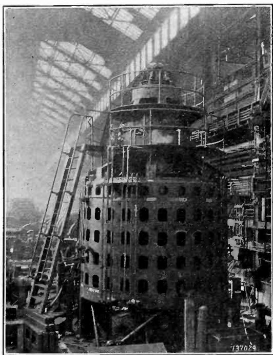
FIG. 6—28,000 KV-A., 11,000-VOLT, 3-PHASE, 50-60 CYCLE, 428-514 REV. PER MIN. VERTICAL WATERWHEEL GENERATOR
