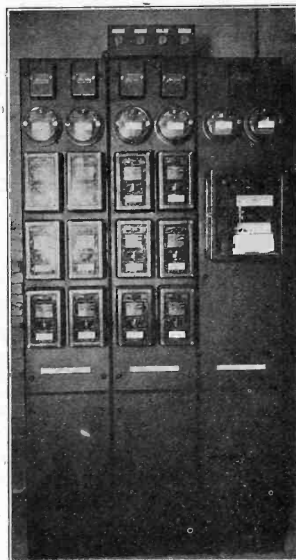
FIG. 6—TYPICAL RELAY PANEL AT RING STATIONS
