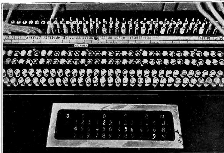
FIG. 23—CALL INDICATOR AT AN INCOMING TRUNK POSITION IN A MANUAL OFFICE
