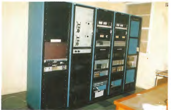
L to R. R.O.E.S. rack, standby program link, 3RN input equipment, 3 LO input equipment, miscellaneous equipment.
