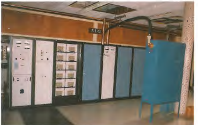
3 LO transmitter with balanced load in foreground.
