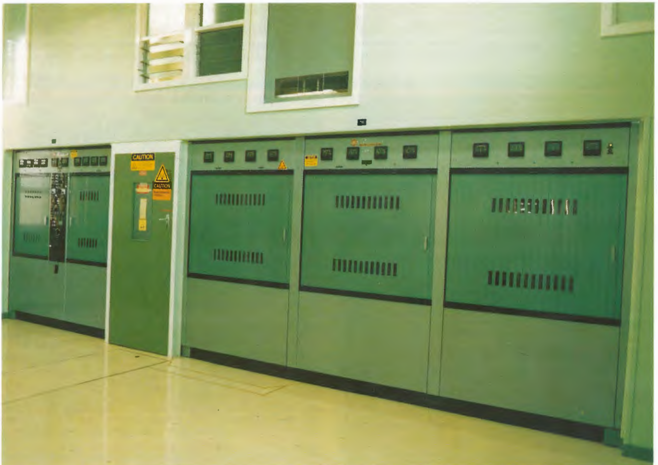
10 kW standby transmitter (L) and 50 kW main transmitter.
