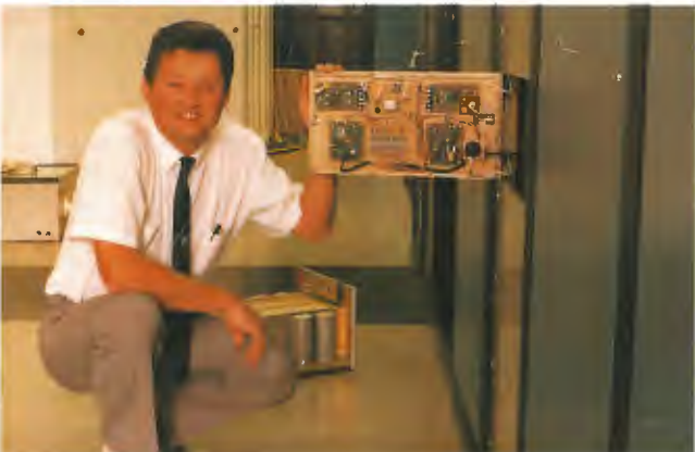
Station OIC Gerd Messig with main and standby RF exciter unit.
