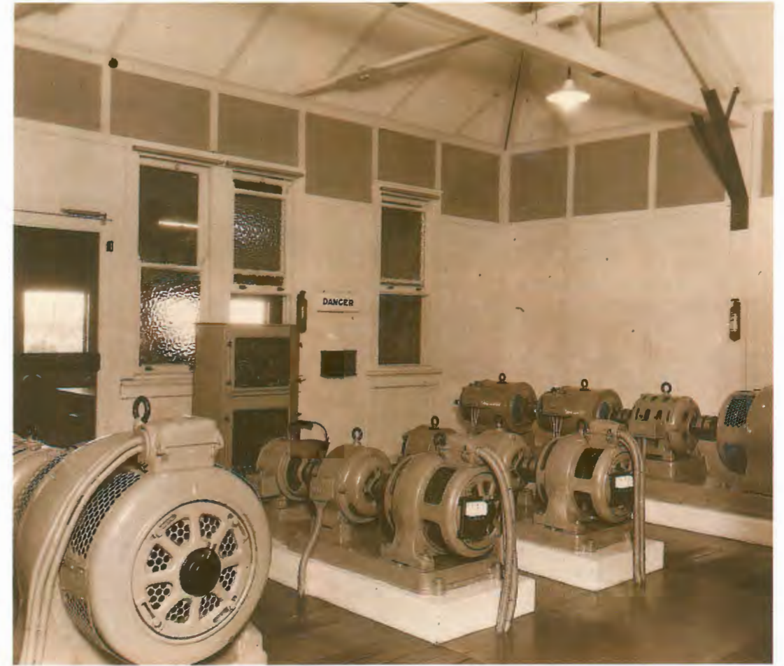
Original transmitter power supply motor-generator sets.
