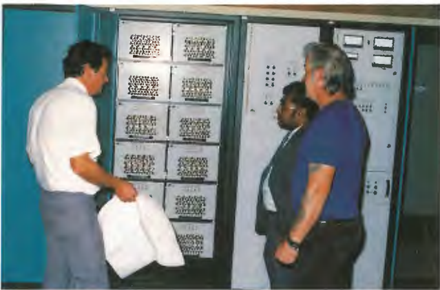
L to R. Station OIC Gerd Messig, Project Engineer Hartley Fernando and Rudy Baranauskas inspecting RF modules.
