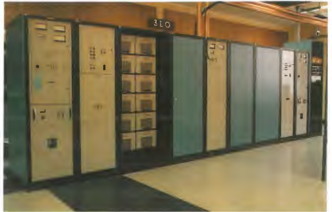
Complete 3LO transmitter comprising parallel 25 kW units.
