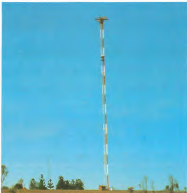
4RK station radiator.
