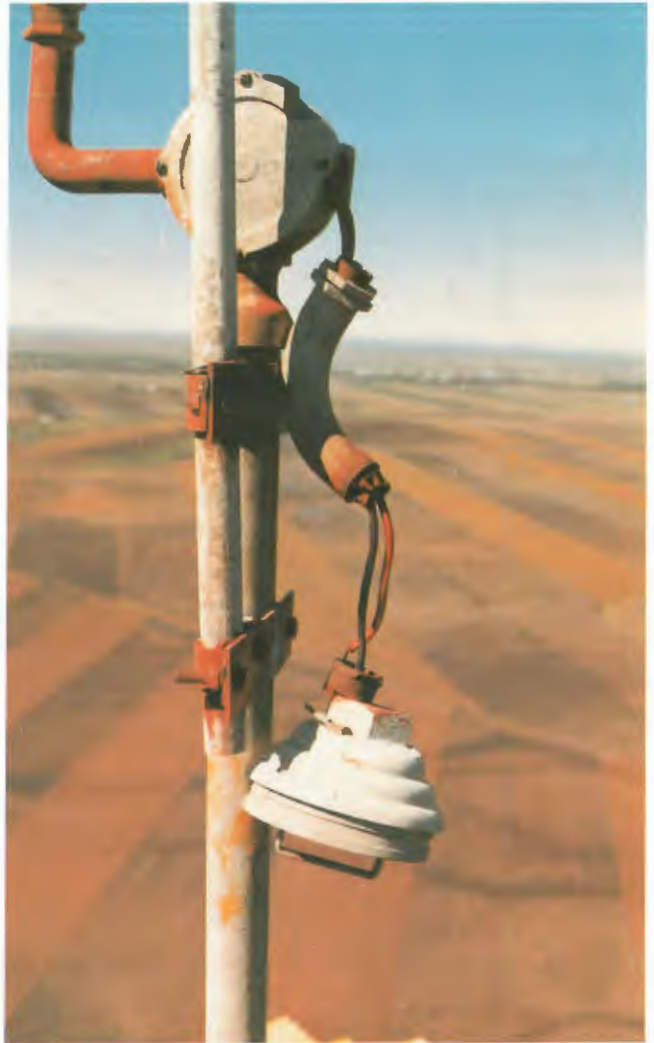
Damaged mast lamp fitting.
