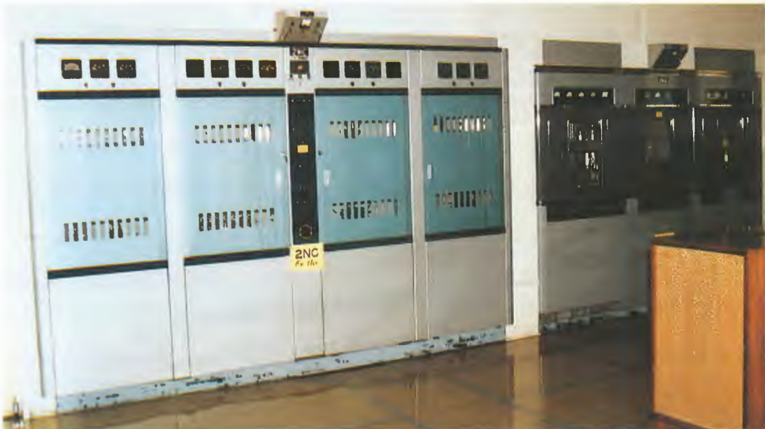
Main transmitter – 10kW on left.
