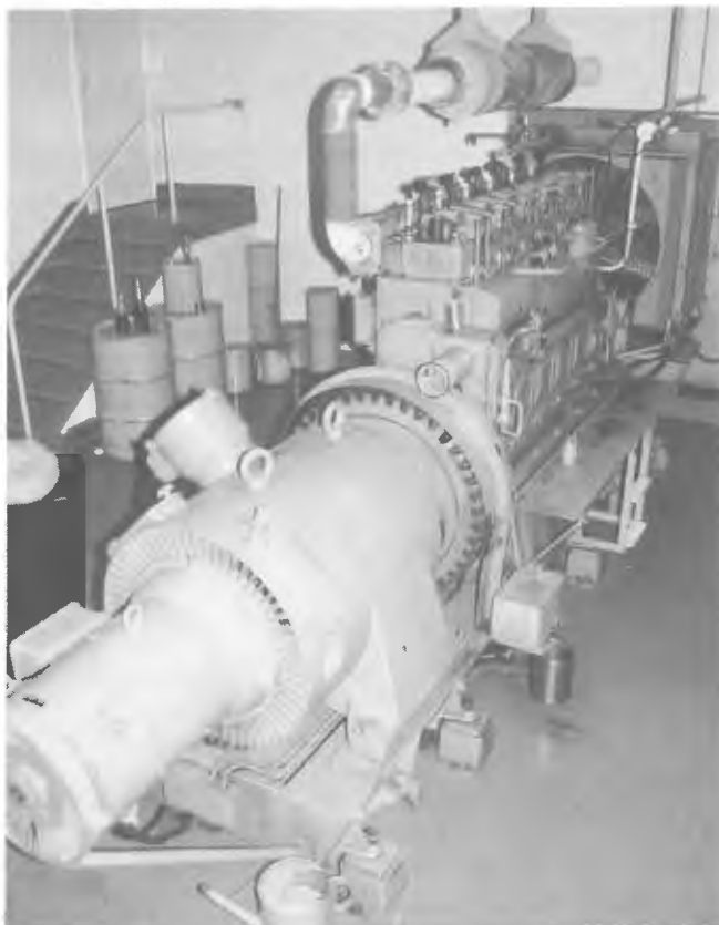
Deutz auxiliary power plant ABT2 Hobart.
