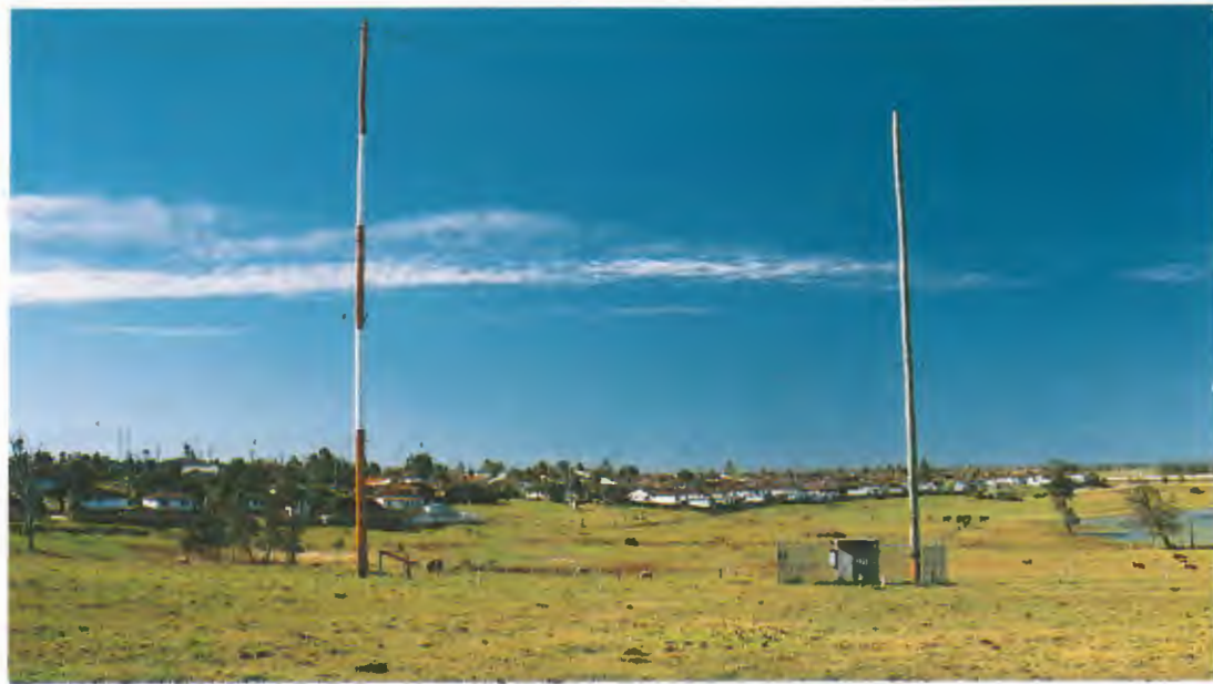
2NC standby radiator.
