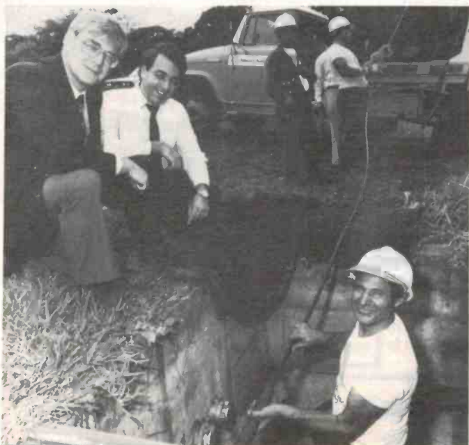
At last. A telecom line crew install the first production fibre link in Sydney.
