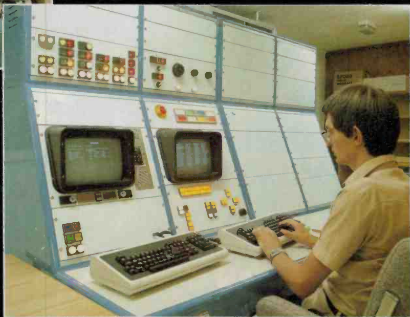
Below. Control console. This is the astronomers' control console. It was designed and manufactured by the ANU's own workshop.
