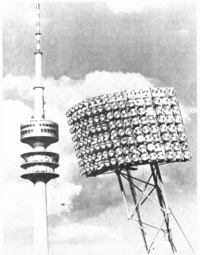
A total of 550 floodlight projectors are used in the main Olympic Stadium. This illustration shows one of the two main towers each with 144 projector units. The total installation draws over 2,000,000 Watts.
