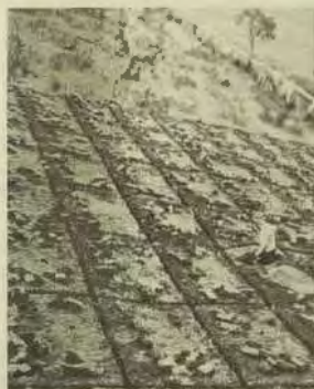
The earth system being laid out. Miles of copper wire crossing and re-crossing and soldered at the joints make it efficient.
