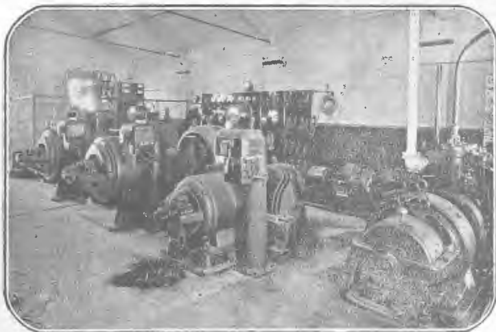
Auxiliary Power Plant at 2FC Station at Pennant Hills, which is brought into operation if the council power fails.
