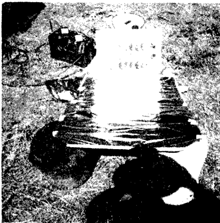
Charge System used. 600 x 300 mm Solar Panel, 1 x 2 metre Foil Covered Plywood Solar Booster, 400 Amp-Hour Battery, 0-5 Amp Amp-Meter, and Multimeter to monitor voltage.
