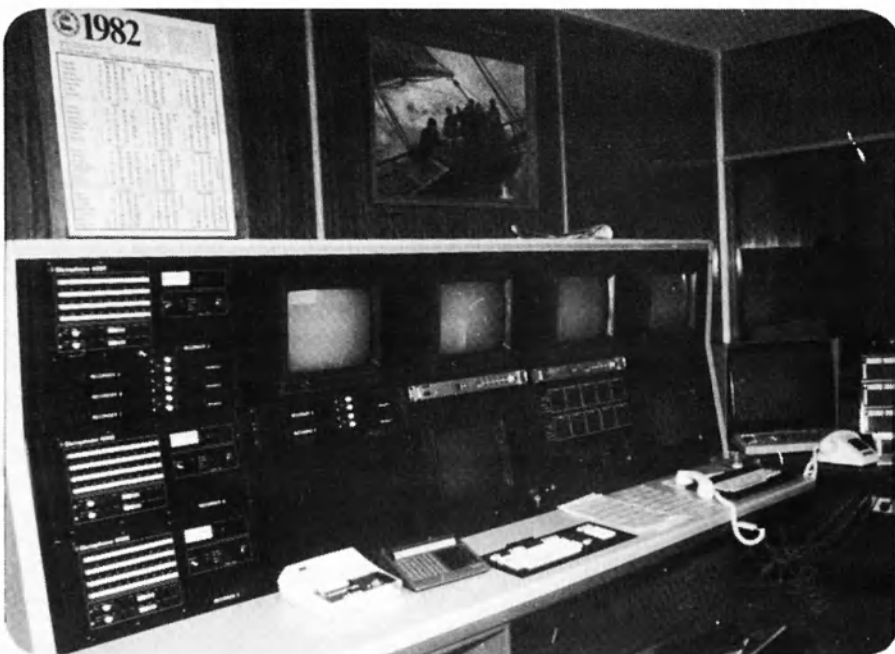
Duty officer's control and monitoring area. Computer and VDU on RH corner of console.
