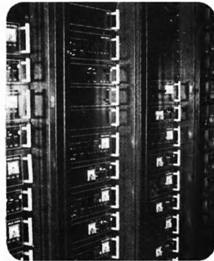
Partial view of the UHF transmitter rack.
