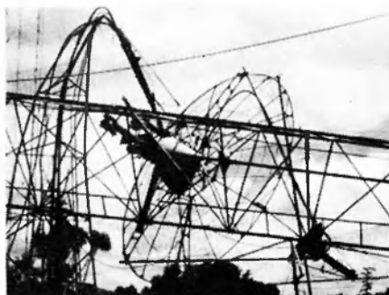
Looking through collapsed tower towards dish.
