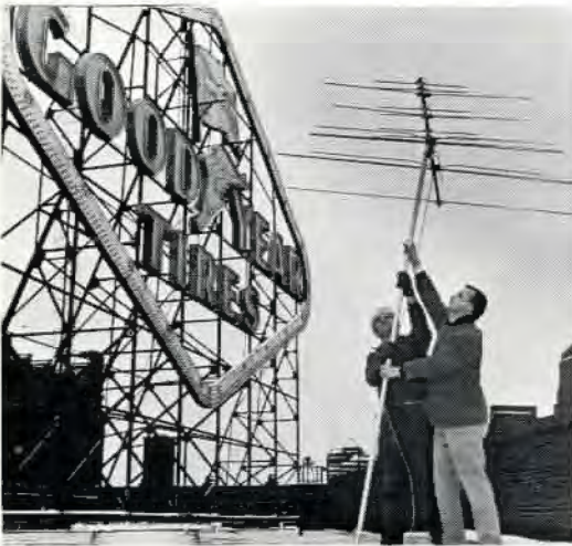
AKRON—Speedy techs Dennis and Clark installed Colorceptor atop Goodyear Theatre at 10:30 A.M. on Inauguration Day
