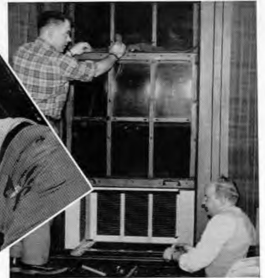
Bill Brey (above) carefully fits weatherstripping into place before sealing window against air leaks. Walt Scheck takes another turn on a retaining bracket
