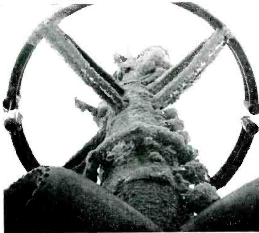
Fig. 21—Ice formation on antenna at Empire State Building. Note the effect from the application of heat to the radiators.
