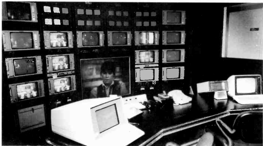
Fig. 6. New York Skypath Control room.
