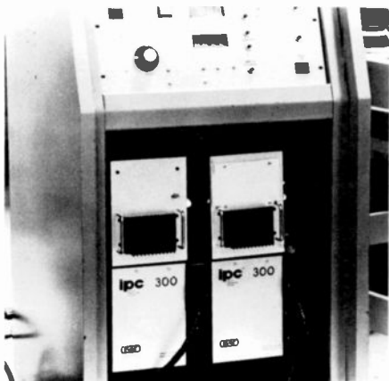
Controls for the multipath segment winder showing the IPC300 microprocessor.
