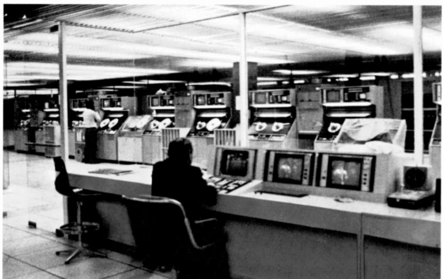
Fig. 6. The VTR editing system, located at the main broadcast center in Buenos Aires, was designed to provide synchronous operation among all of the tape machines.
