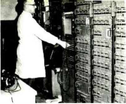
Fig. 7 — Monitoring performance of frequency division cable multiplexer.
