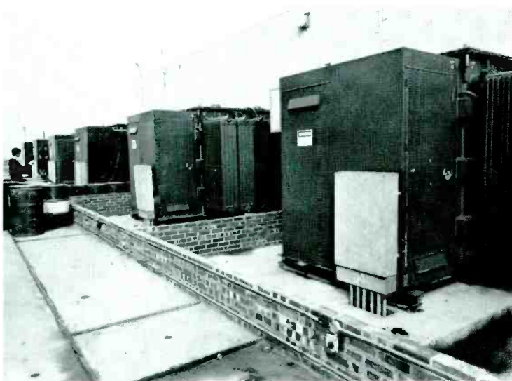
Fig. 7 — High-voltage DC power supplies.
