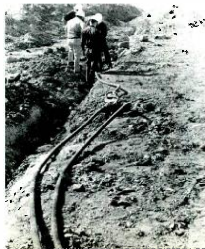
Fig. 6—Armored cables and "Y" splice case.
