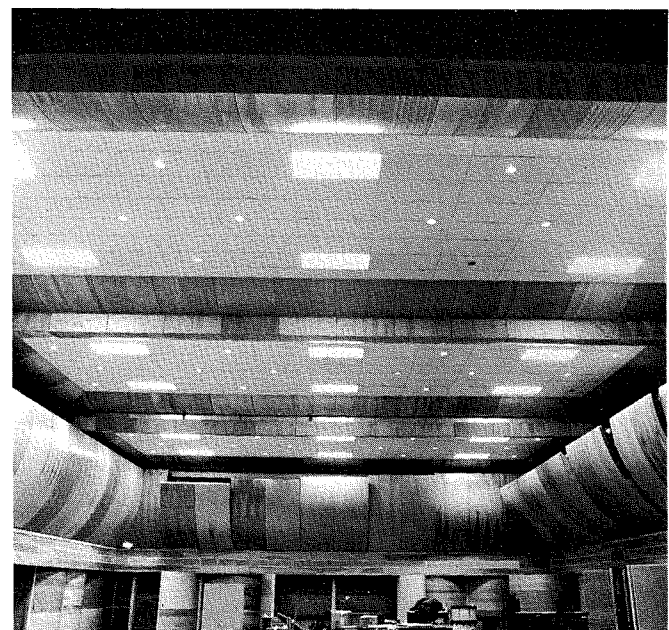
Fig. 11—One of the many combinations of adjustment possible with the three types of adjustable acoustical elements in the main portion of Studio A. These include the ceiling stepped, the middle wall panels staggered, and the wainscot panels opened at random.
