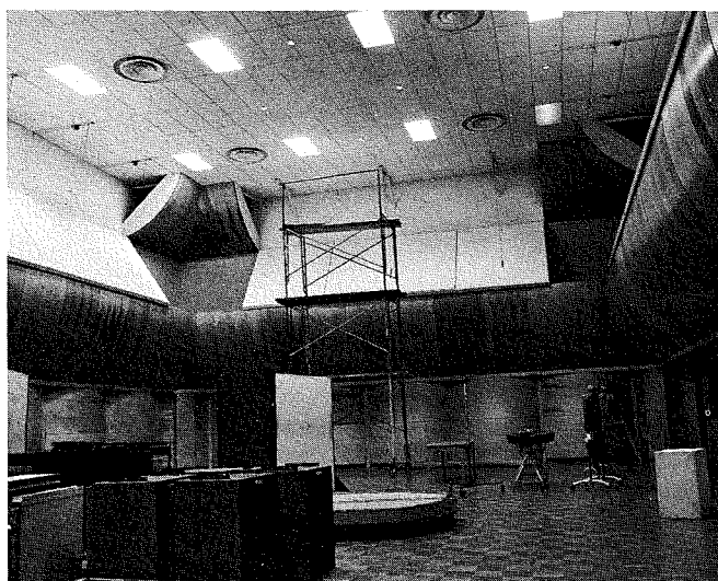
Fig. 14—General view of the studio with the uppermost hinged ceiling corner panels lowered, completely exposing the absorptive backside of the panels.
