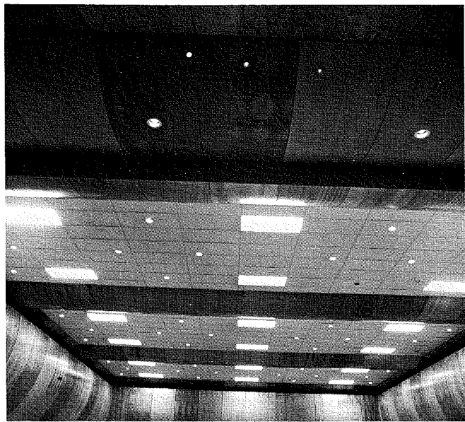
Fig. 9—Studio A ceiling at minimum height.
