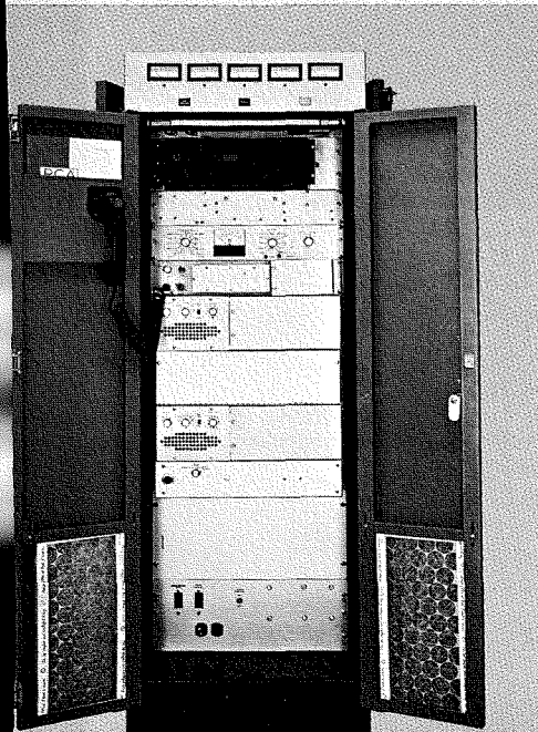
7—Complete rack-mounted base station equipment.
