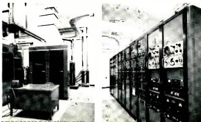
Fig. 6—Views of left and the right portion of a room in the central building containing operating positions, array of control racks, and driver units.
