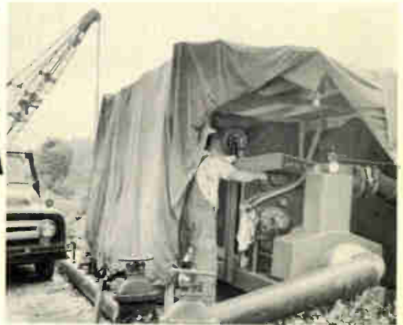
9:15 A.M. SPARE GENERATOR IS ON THE JOB.
