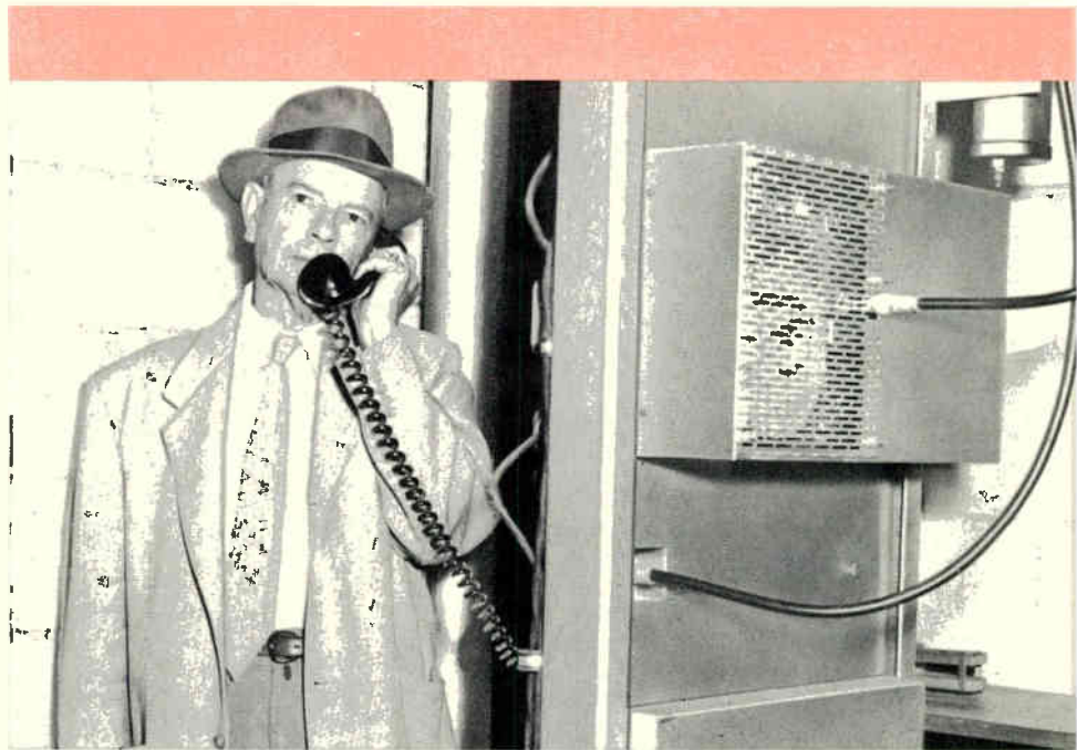
Fig. 8—L. G. Wainman, Superintendent of Communications, contacts distant microwave station on service channel handset.
