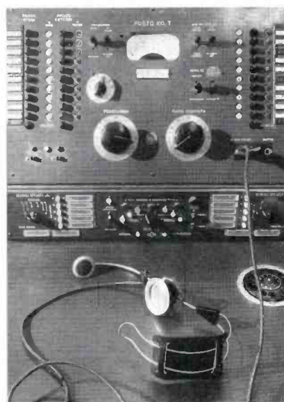
FIG. 20. Close-up of one of ten control panels in master control console. This is the Portuguese position.
