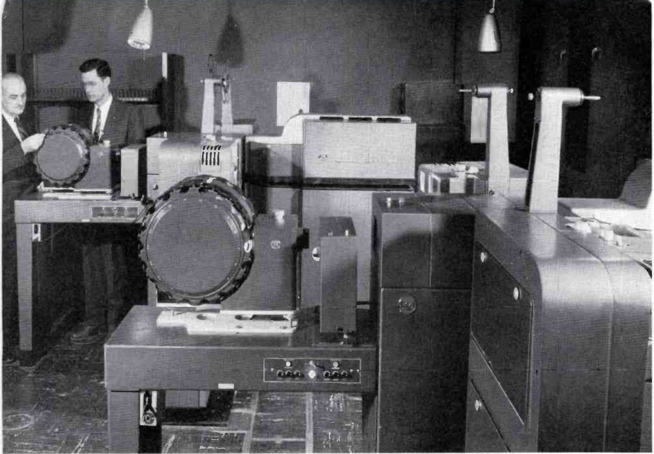
FIG. 30. WBTB's film room contains two RCA 3-V Color Film Cameras, four TP-6C Film Projectors, two TP-7A Slide Projectors and two Chromascan units. Space has been reserved in this room for future installation of color video tape equipment.
