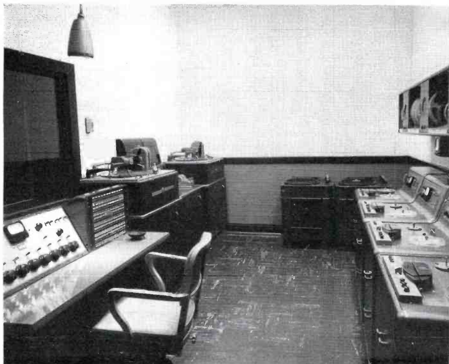
FIG. 48. Interior of the WBT recording room. Control console, at left, faces into Studio C and may be used to control a program originating in this studio independent of master control.
