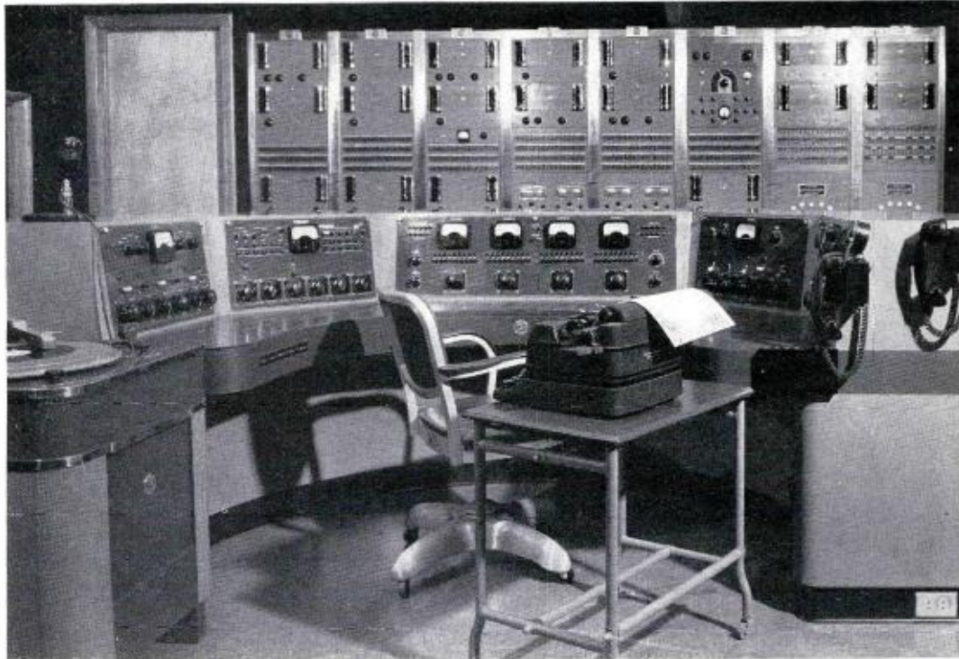
FIG. 10. Radio master control viewed from lobby.
