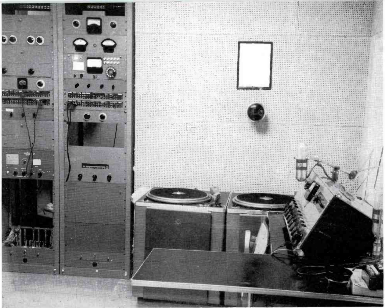
FIG. 3. Complete equipment facilities in Control Room A include a BC-2B Consolette, two BQ-2A Turntables and two equipment racks.
