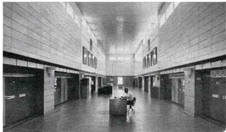
FIG. 12. At the transmitter center in Portugal 13 broadcast transmitters are used to beam programs to target countries. Shown here is the main transmitter hall housing eight RCA 50-kw transmitters.
