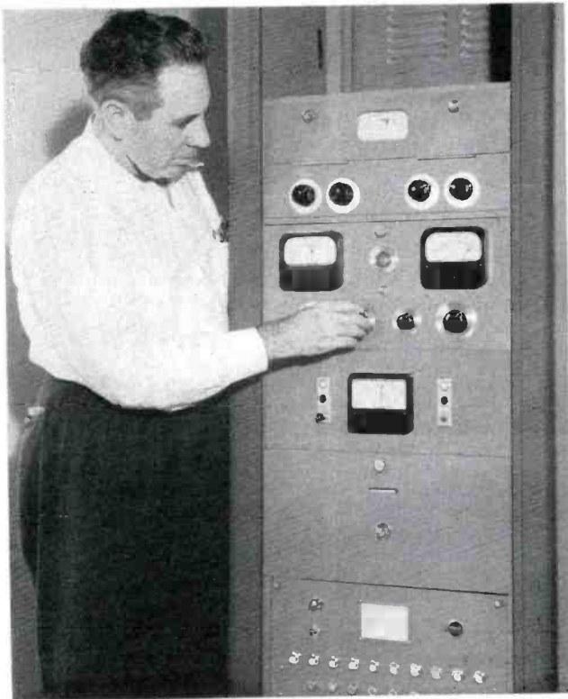
FIG. 9. W. D. Cousar, who maintains all equipment at WHER, checks readings at switching unit of remote control system in transmitter building.
