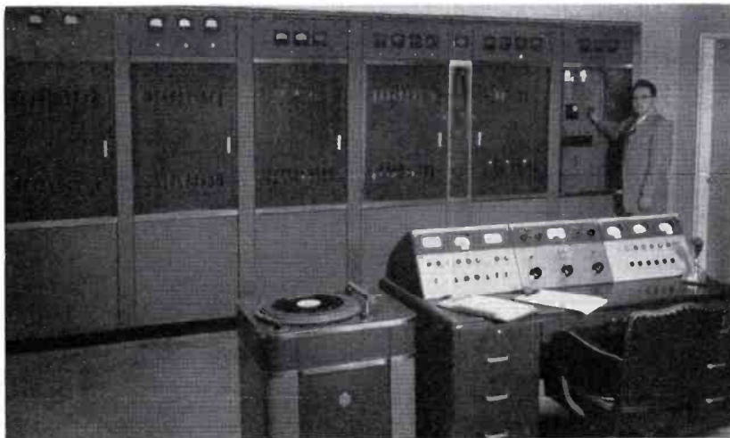
FIG. 5. View of BTA-5H AM transmitter and console. Two cabinets at left are phasing equipment. Right-hand console turret contains control for switching each of the three AM transmission lines to a spare line. Engineer in picture is B. J. Weimer, Transmitter Supervisor.
