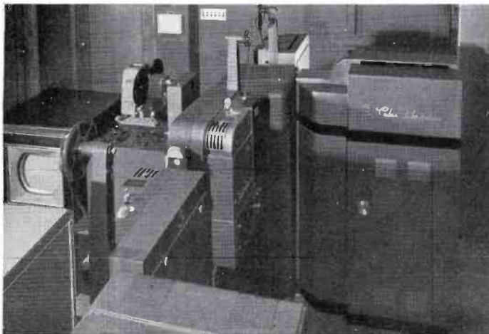
FIG. 17A. View of WISH-TV projection equipment. In foreground, TK-20D iconoscope camera. In background, TP-3 slide projector, TP-15 multiplexer, and TK-26 3-V color camera.
