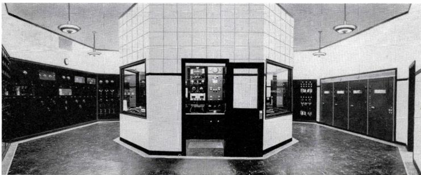
FIG. 1. Interior of transmitter building at KSTP looking toward the rear of the octagonally shaped room. At the far right, the four cubicles of the BTA-50G 50 KW AM Transmitter can be seen. Just to the left of the BTA-50G is a composite 1-kw stand-by transmitter housed in two cabinets. The control room at the center of the main transmitter room contains the transmitter test and measuring equipment as well as facilities for programming of records and station breaks. At the left of the control room, a portion of the old composite 50-kw AM transmitter can be seen. This composite 50-kw unit takes up approximately one-half of the wall space of the transmitter room. In contrast to this, the new BTA-50G occupies less than 15 feet of wall space—an area formerly occupied by a 10-kw FM transmitter.
