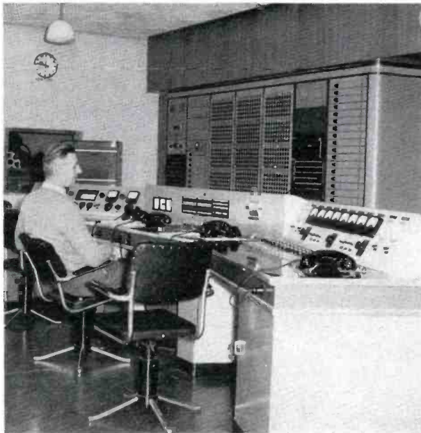
FIG. 10. Master control at Munich Studios feeds program signals to transmitters for target countries. (This unit was designed and built by RFE engineers.)
