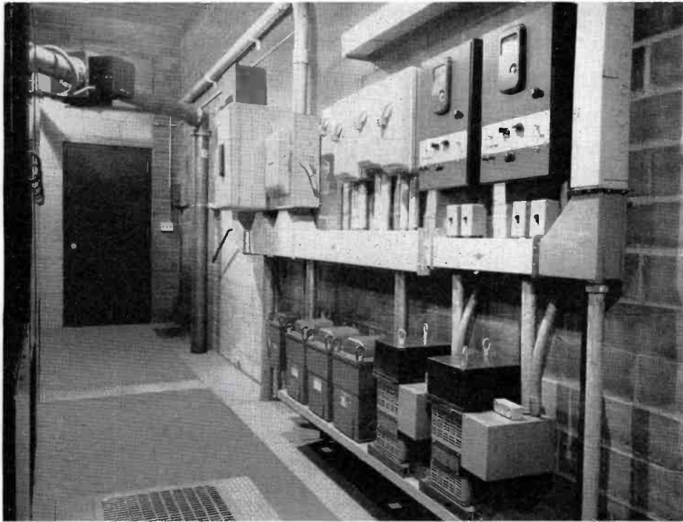
FIG. 6. KSTP chose to modify the typical arrangement of the wall-mounted switch gear—frankly, we feel that they have improved the arrangement. In the typical layout, the distribution transformers are mounted at the upper right at eye level—KSTP has installed all heavy components at floor level which eliminates the necessity for reinforcing the tile wall. Starting at the upper left, the top of the main line 400 amp/600 volt disconnect switch can be seen. This is the only piece of switch gear which must be supplied by the customer. Next in line is the plate breaker, a Delta-Wye switch, and the low-power, intermediate and distribution breakers. The two units to the right are the contact making volt meters for the two voltage regulators at floor level. The three transformers to the left are the 460/230 volt distribution transformers which supply regulated voltage to the filament control circuits. The door to the rear gives access to the transformer vault and is interlocked for personnel protection. The clear layout is typical of the sound engineering practices used at KSTP.
