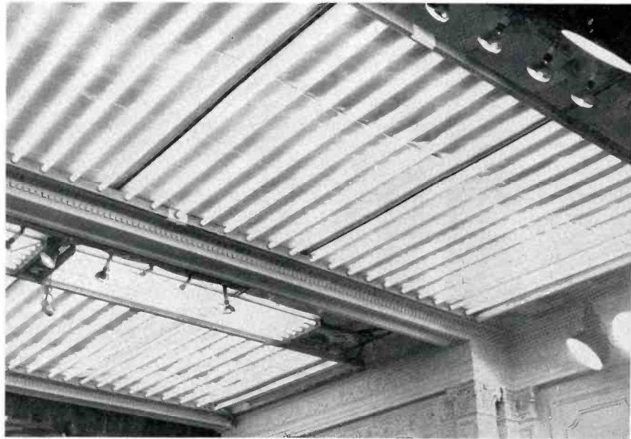
FIG. 22. Partial view of Studio "A" fluorescent lighting banks. Fluorescent lights are used here to provide an even overall lighting for the chapel interior. To get the correct color balance for films, "White" and "Warm White" tubes are used alternately in the lighting sockets.
