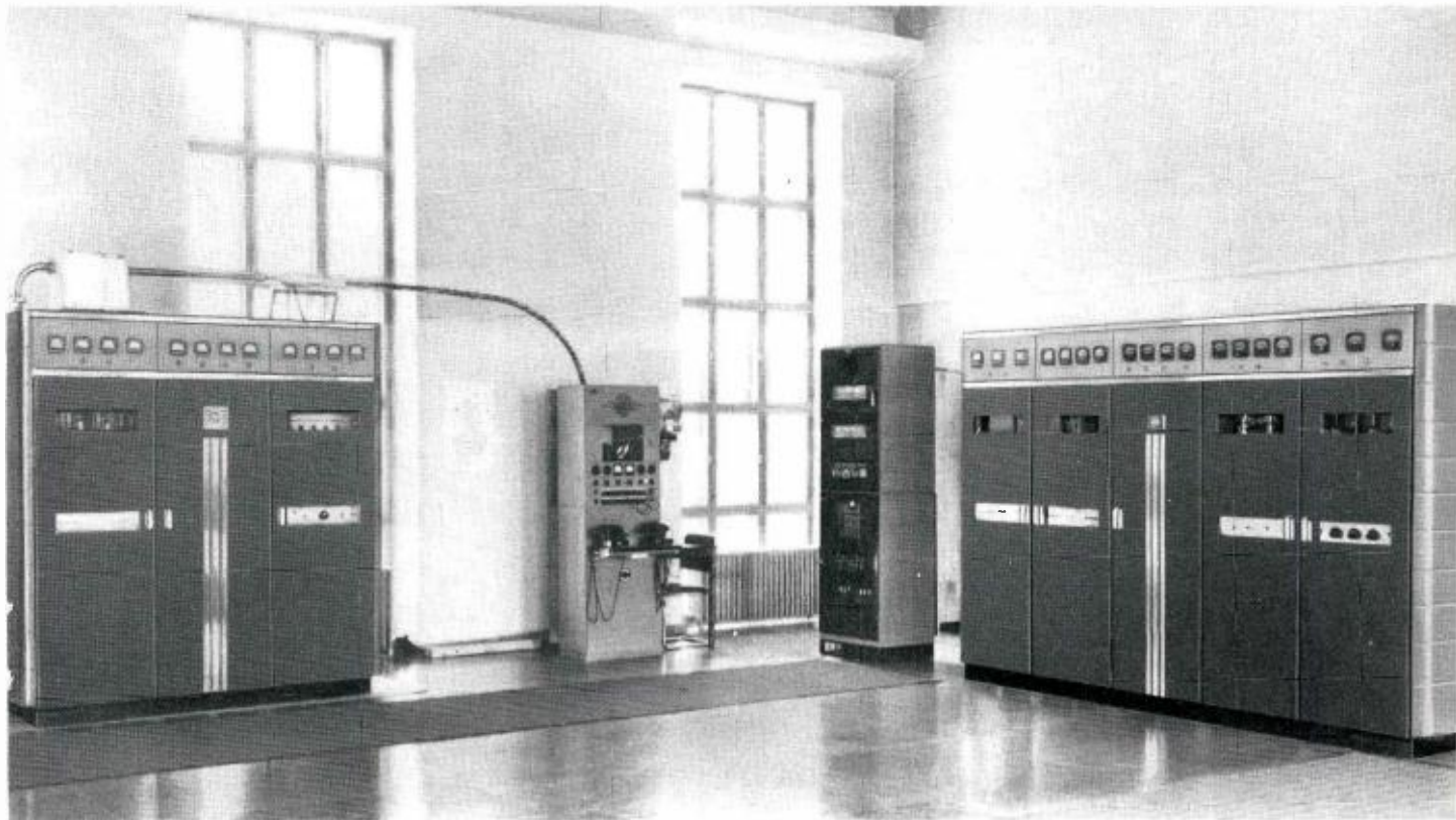
FIG. 2. Lahti station has one BTF-3B and one BTF-10B FM transmitter (right).
