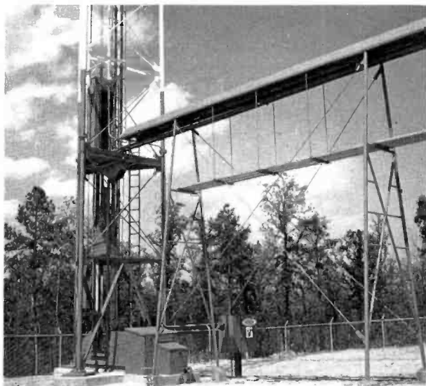
FIG. 6. Part of 80-ft run of transmission line running from tower to building. Inverted V-type steel cover plate protects line from falling ice.
