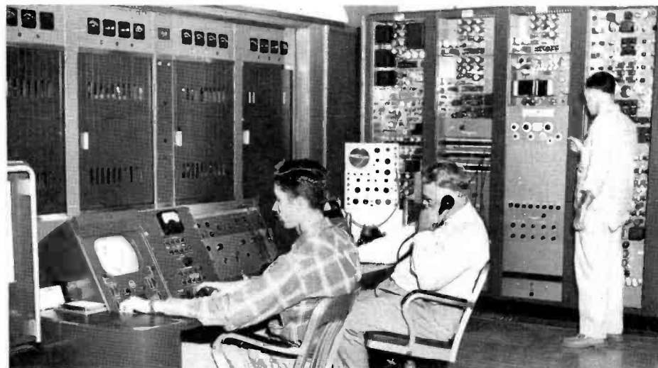
FIG. 5. Operators' control console located directly in front of RCA TT-50AH 50-kw transmitter. Standby 2-kw transmitter is also in this room.
