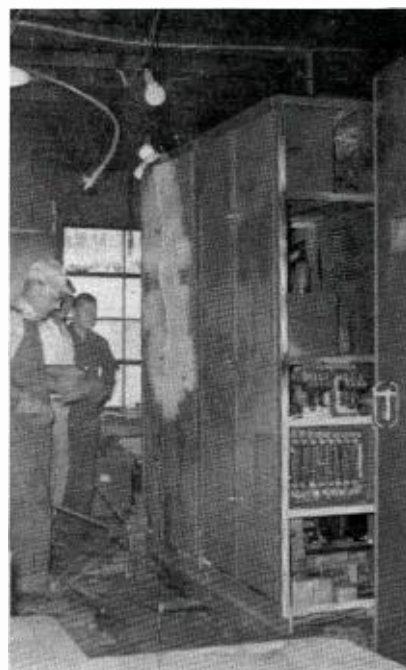
WHBL fire damage in transmitter building. Adjacent RCA FM transmitter, shut off during fire-fighting, returned to air in less than one hour.
