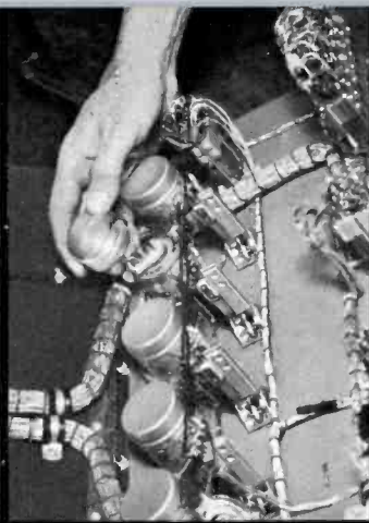
Every component is easy to get at for inspection and maintenance.
