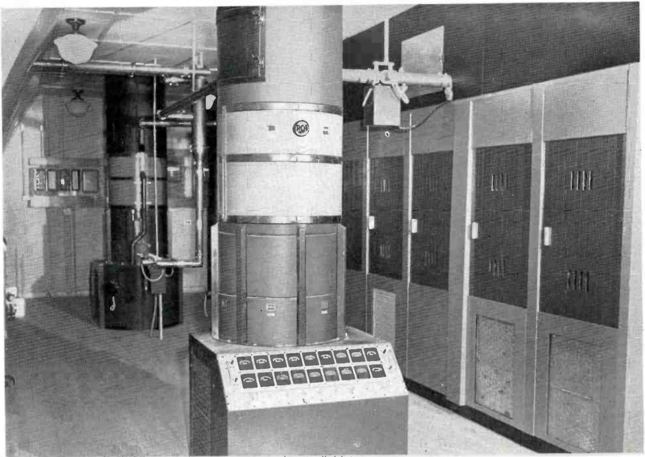
FIG. 6. Shown is a front view of the KBTV 25-KW Aural Power amplifier.
