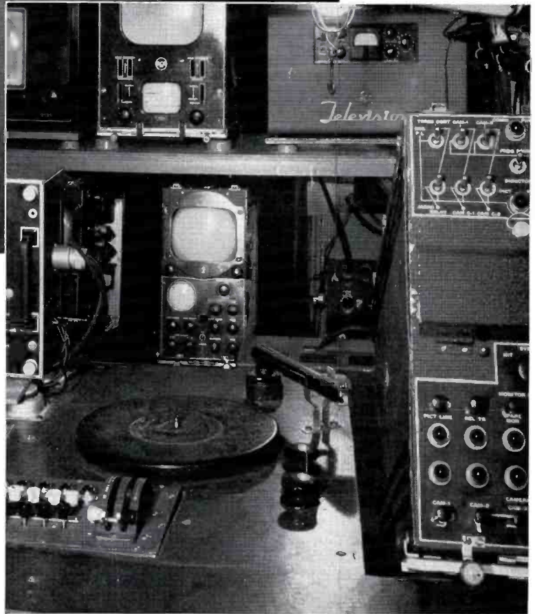
FIG. 16. Close-up view of a portion of the TV Mobile Unit showing the "Director-Audio Control" equipment.
