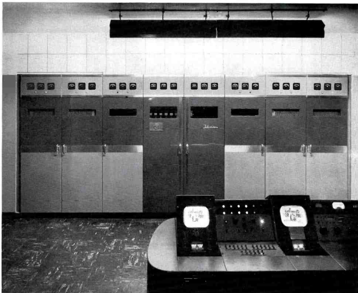
FIG. 18 (above). Front view of the neat, flush-mounted arrangement of the WDSU-TV, RCA TT-5A Transmitter.
